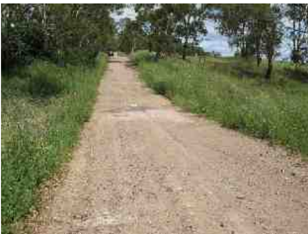
PLATE 23 Waterloo Rd, damaged causeway at 7.7 km.
