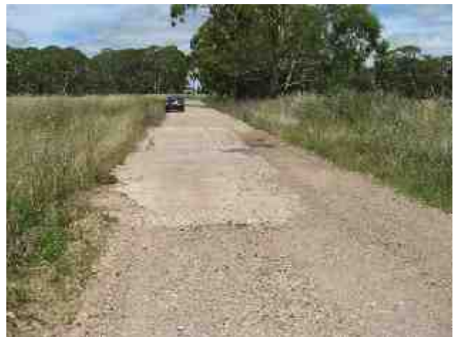
PLATE 28 Waterloo Rd, Damaged causeway at 9.0 km.
